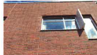
Brick broken at lintel - west exposure
