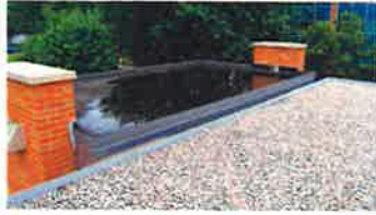
Main entry roof canopy Roof over the main entry canopy is a single ply EPDM roof. The slope is inadequate so ponding occurs. When this roof is replaced the slope to scupper drains should be corrected.
