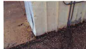
Metal panel bottom rust
