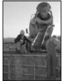
Concrete is poured for the foundation walls of the three-story academic wing of the new middle school.
