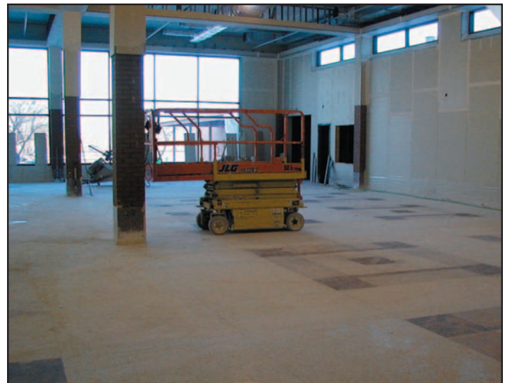
Next to the ninth grade center, construction continues on the new commons/cafeteria (shown here). On the east end of the school, the new fieldhouse is being built.
