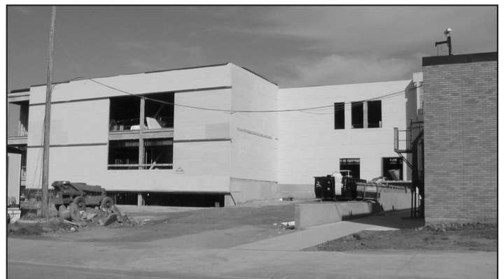
Additions at Moorhead High School include a ninth grade center, commons/cafeteria, a fieldhouse for physical education, and a scene shop addition to the theater. The three-story ninth grade center shown here will create smaller learning communities for ninth-graders and ease the transition to high school.
