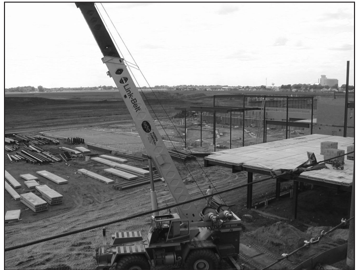
▲ Above: From the third floor of the middle school's academic wing, the areas where the media center, music classrooms, cafeteria and gymnasium are under construction can be seen.
