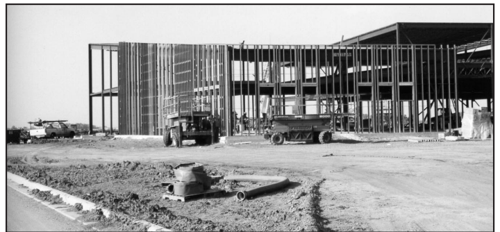
Structural steel and metal stud framing have been erected for the new K-5 elementary school in south Moorhead. This portion of the school is now being bricked.
