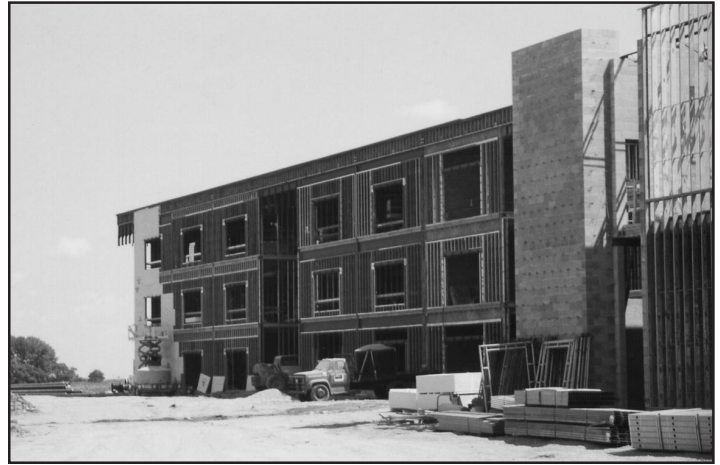
The three-story academic wing of the new middle school is being enclosed. Students in grades 6-8 will attend the new middle school beginning in the 2004-05 school year.
