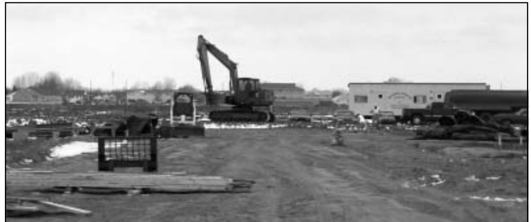
Site work and foundation work, which began Oct. 7, 2002, continue at the site of the new middle school.
