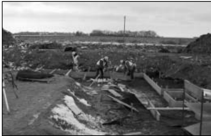
Approximately five weeks after beginning work at the middle school site, workers complete forms in preparation of pouring concrete for the foundation of the school's three-story academic wing.
