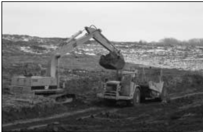
Heavy equipment hauls soil out of the area on the middle school site where the retention pond will be located.
